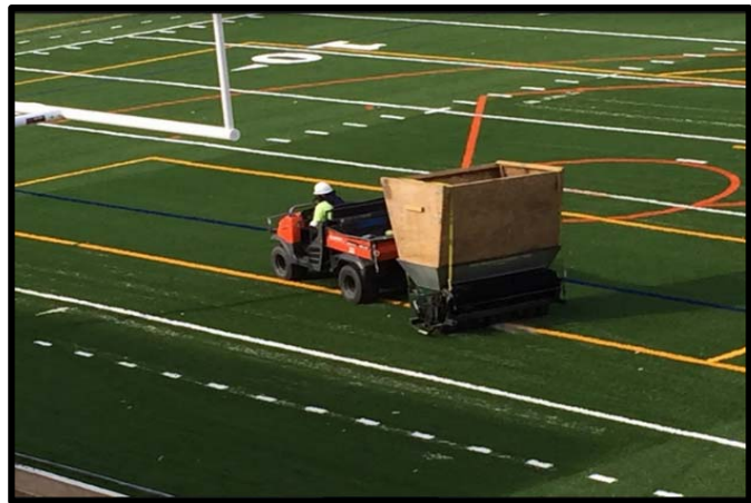
Figure 5: Tire crumb rubber is placed on a field in layers during installation (USEPA, 2016c)
